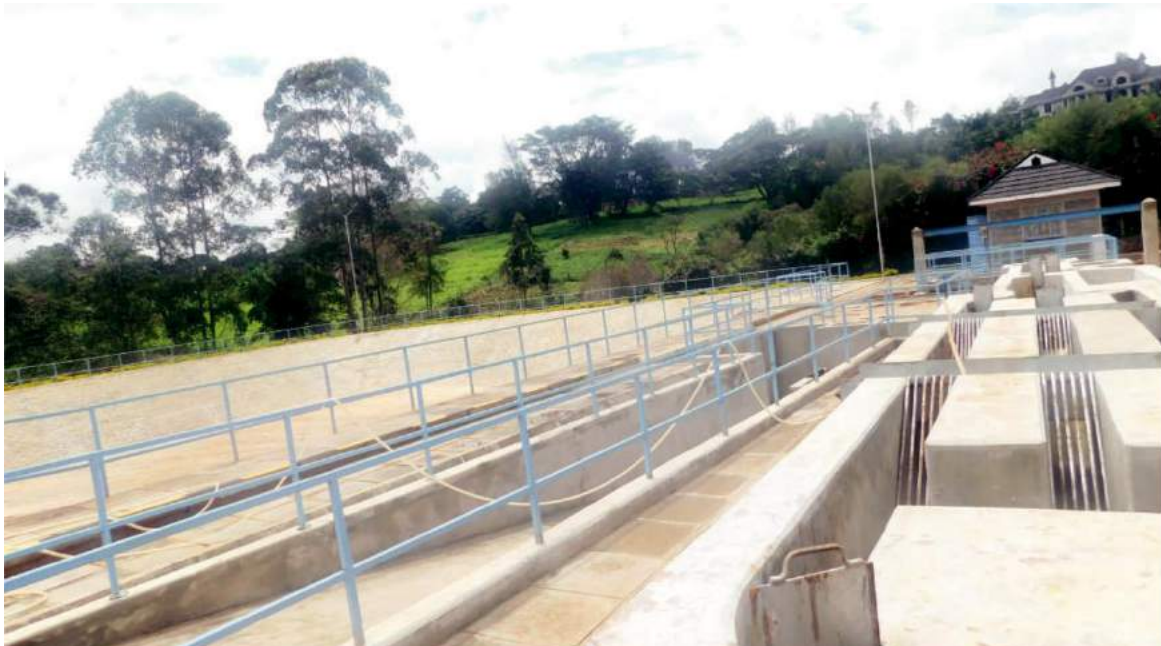
King'ong'o Pumping Station
