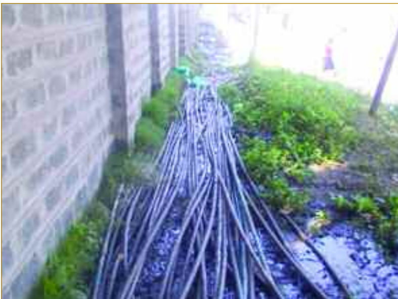
Spaghetti pipes lead to high UfW.
